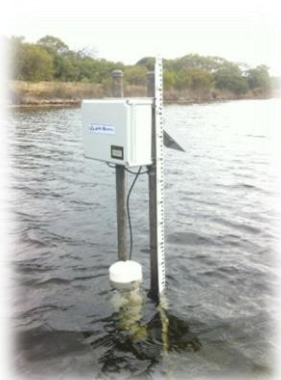
UniData Telemetry Enclosure
