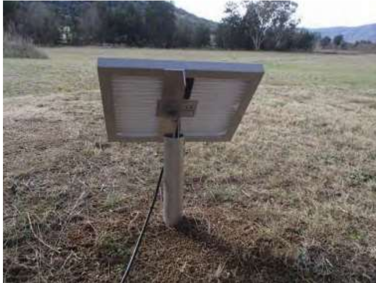
Photo 8: SPPM installed directly in the soil to mount and position a SP22 22W solar panel.
