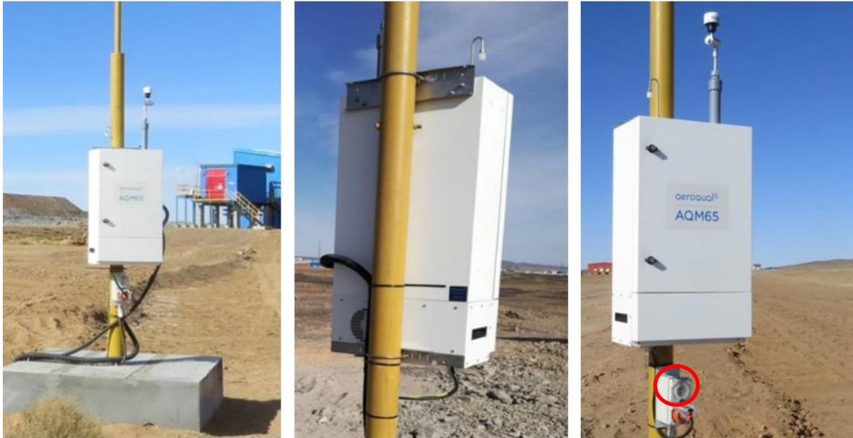
Figure 3 The AQM 65 is mounted to a pole, an additional power point is added to allow a laptop or Aircal 1000 calibrator to be plugged in.
