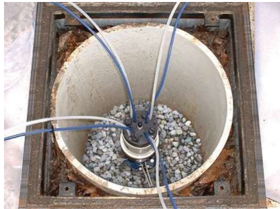
Figure 9-1 Tubing Organized Around the Wellhead
