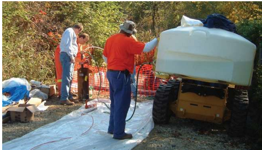
Figure 8-1 Adding Water to the System
